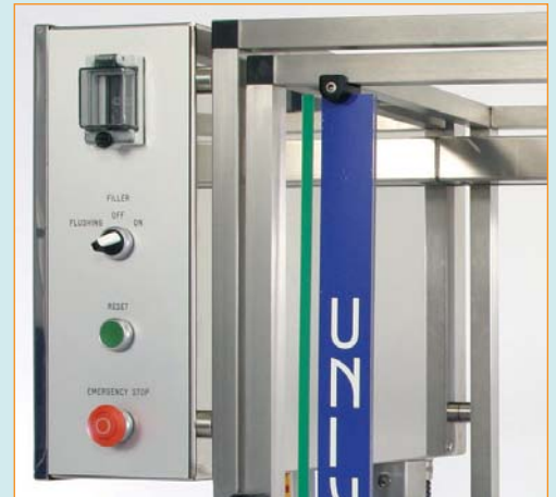
Close up of control cabinet
